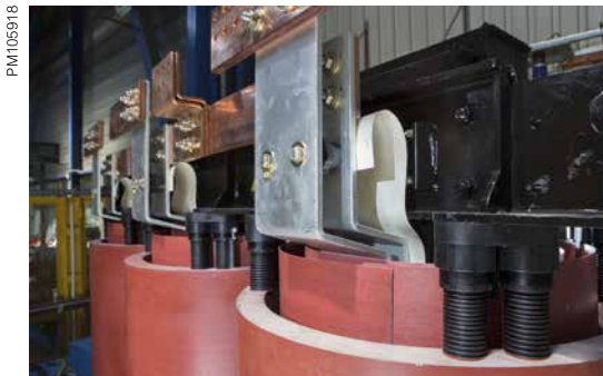
HV coil support wedges
